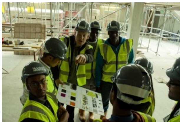
Poplar HARCA Youth Empowerment Board Members are being shown plans of the under construction youth centre. Courtesy: Poplar HARCA
