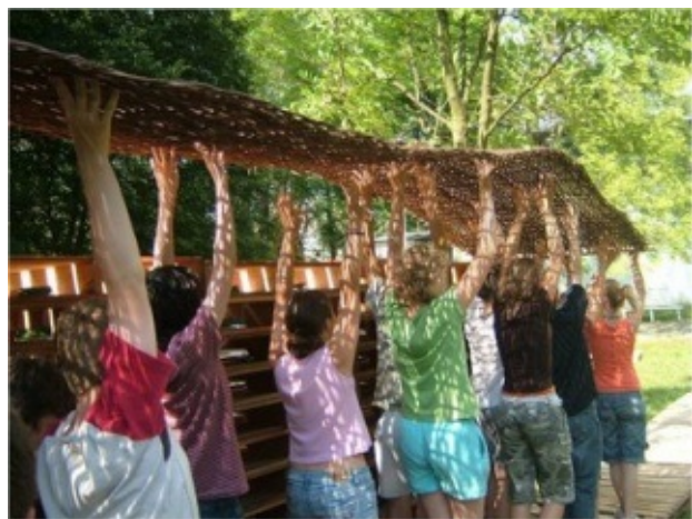
Participants erecting the seven metre long wicker canopy. Courtesy: Gary Johnson (photographer)
